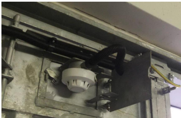
Fig. 11: Smoke detector fitted inside the hatch on substation door.
