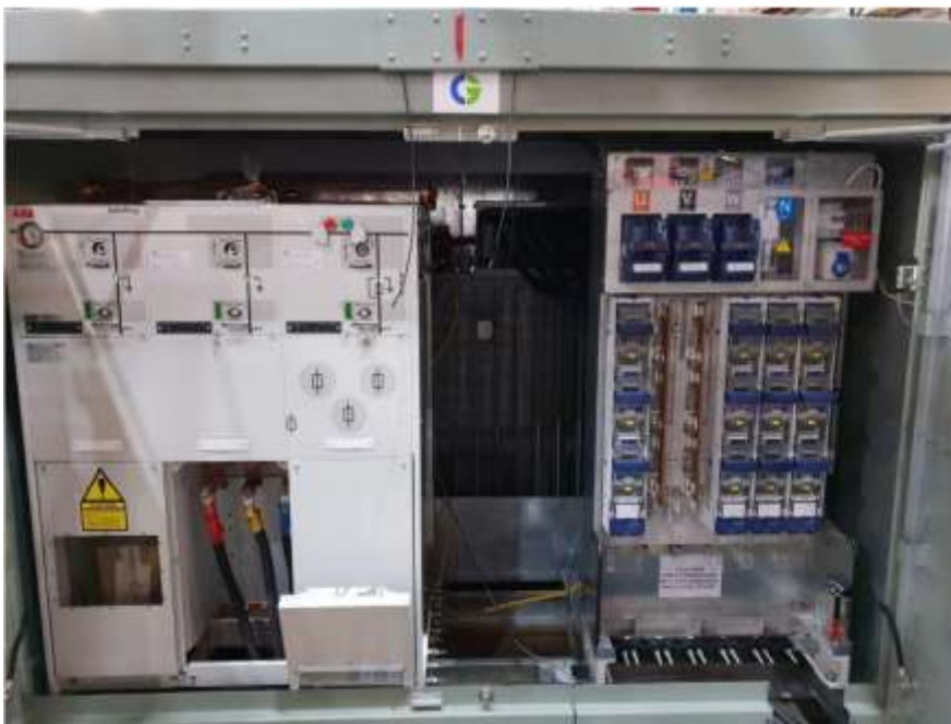
FIGURE 2: UNIT SUBSTATION. SUPPLY ON RMU AND LV PANEL SHORTED OUT
