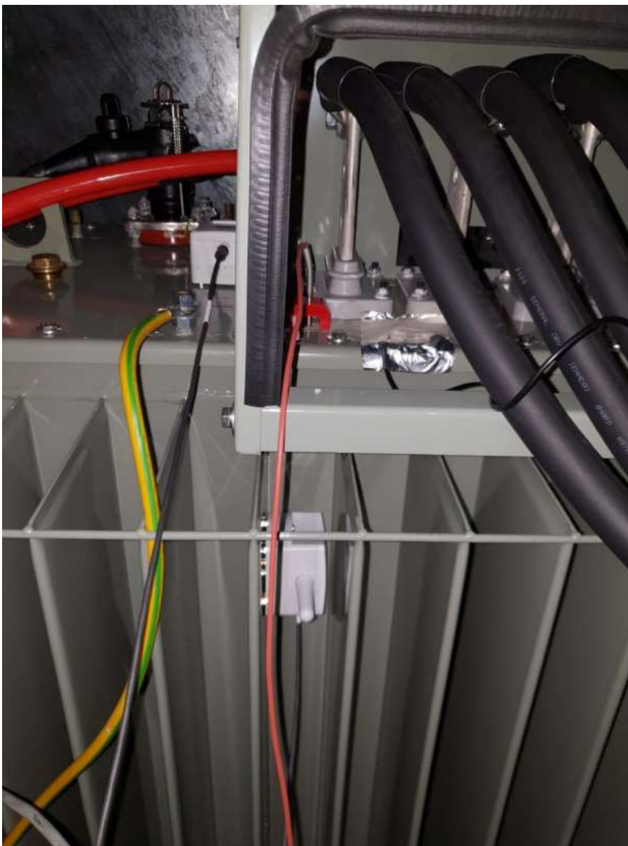
FIGURE 3: PLACEMENT OF TEMPERATURE SENSORS ON TRANSFORMER
