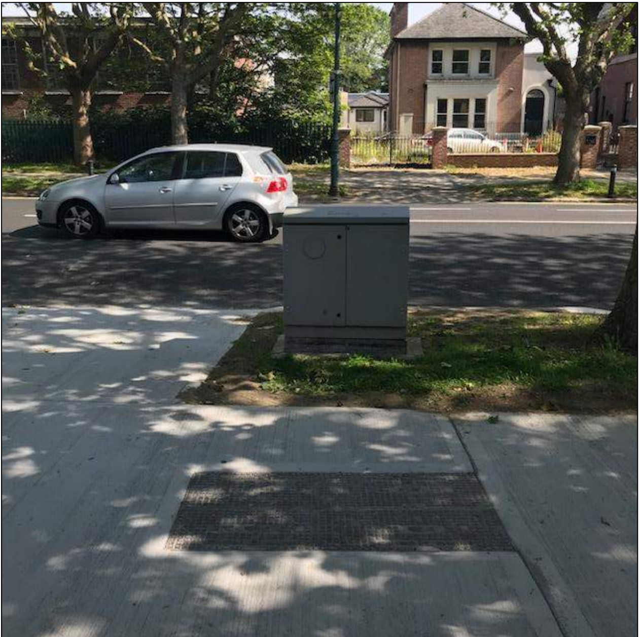
Photo 5: Approx 90m east of leak point. Kiosk location adjacent to ESB cable.
