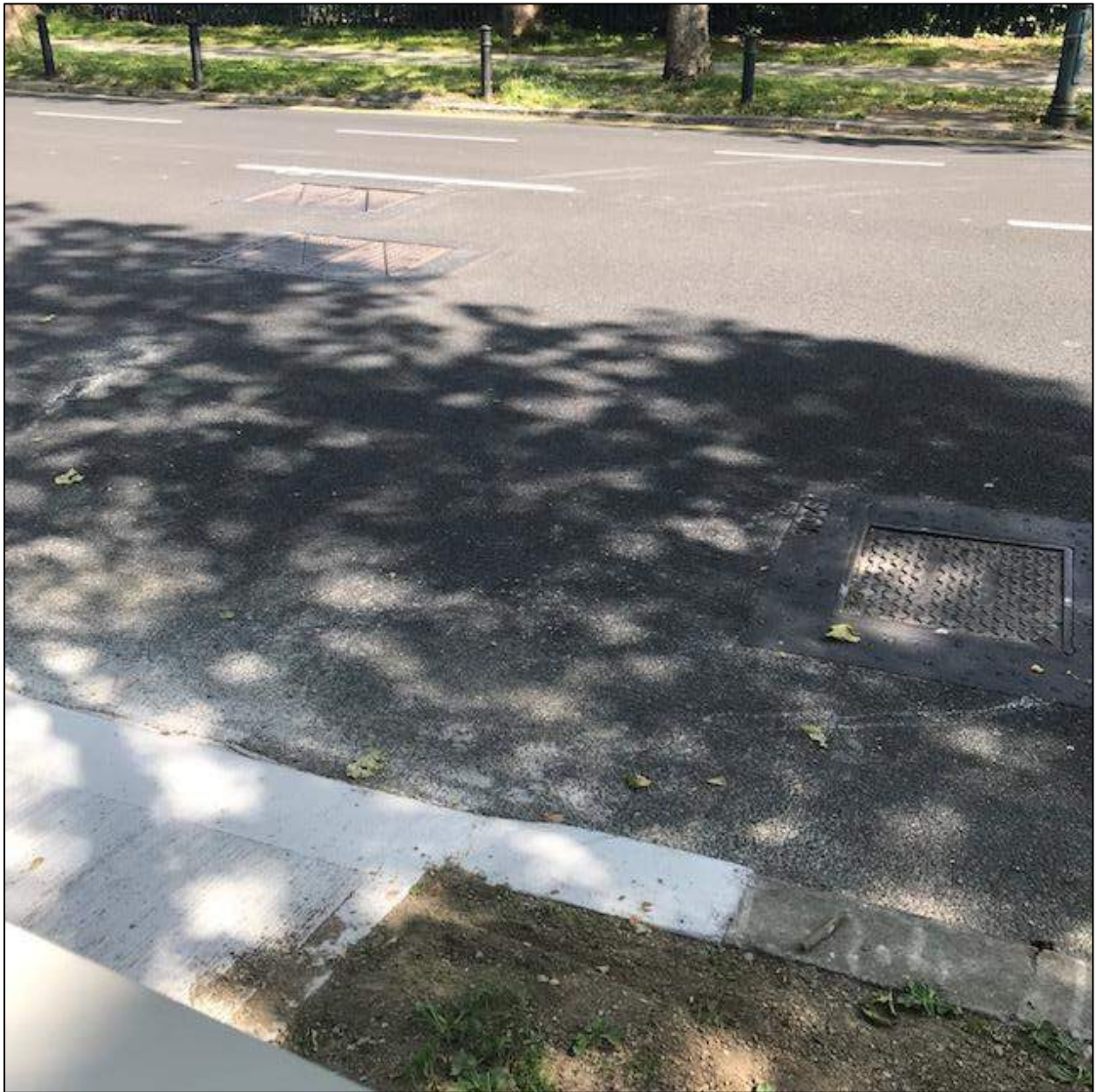
Photo 4: Approx 80m east of leak point. Abundant services on roadway next to ESB cable. Layby area available on the roadway verge for car parking.
