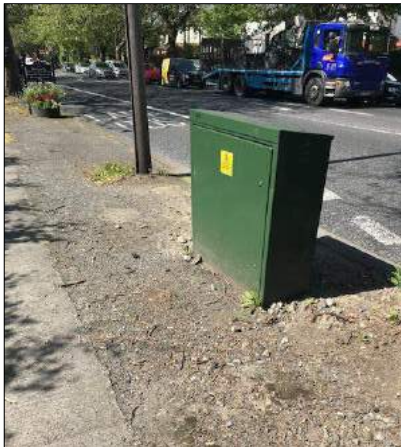
Photo 7: Green Kiosk approx. 180m east of leak point located on Drumcondra Road Upper near southern branch of ESB Cable
