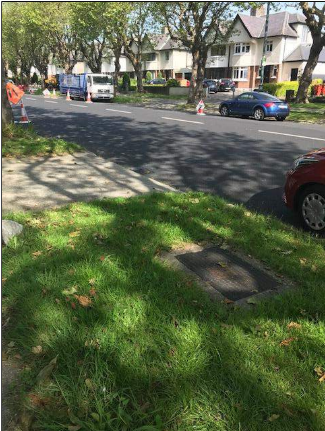
Photo 1: Approx 180m east of Leak Point - View to west. UPC services on grass verge
