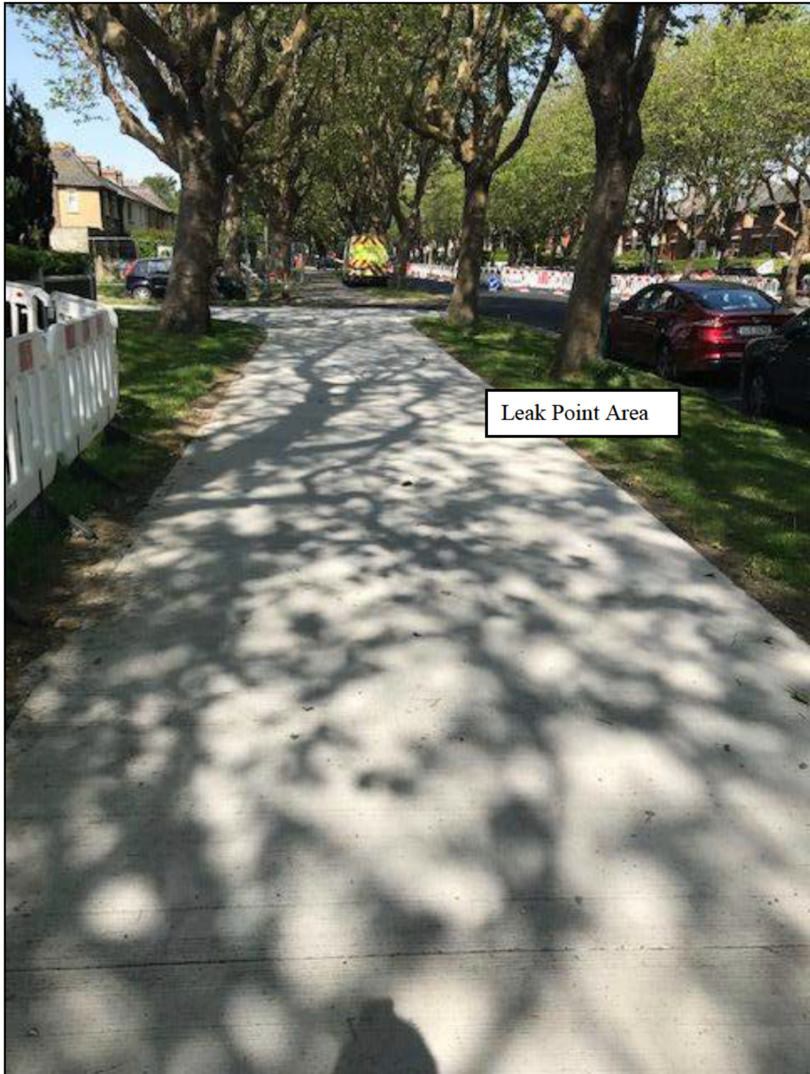
Photo 2: Leak point location in area next to new concrete footpath – abundant services in area
