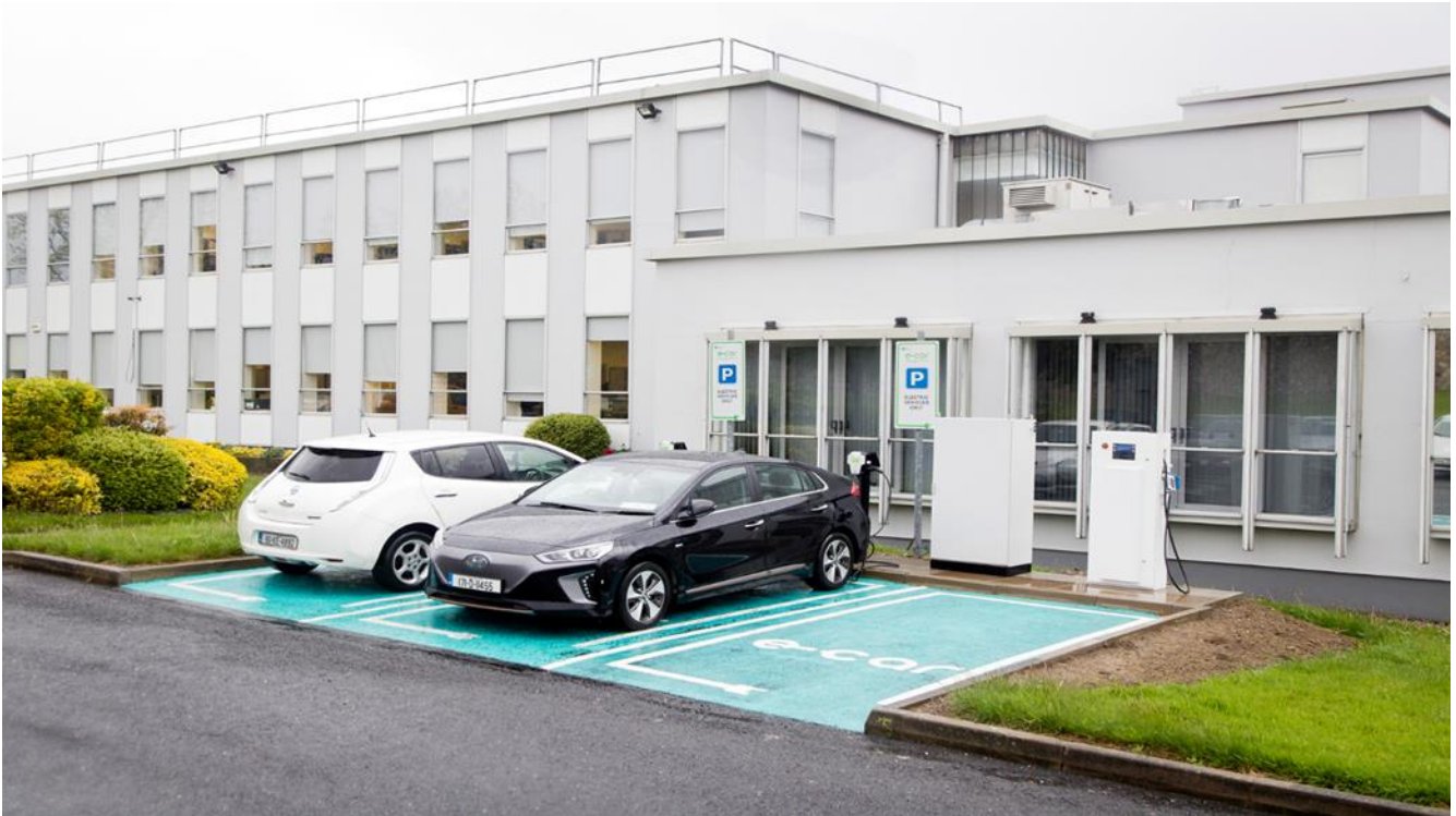
FIGURE 2: IRELAND'S FIRST V2G CHARGING SYSTEM, LEOPARDSTOWN, CO. DUBLIN
