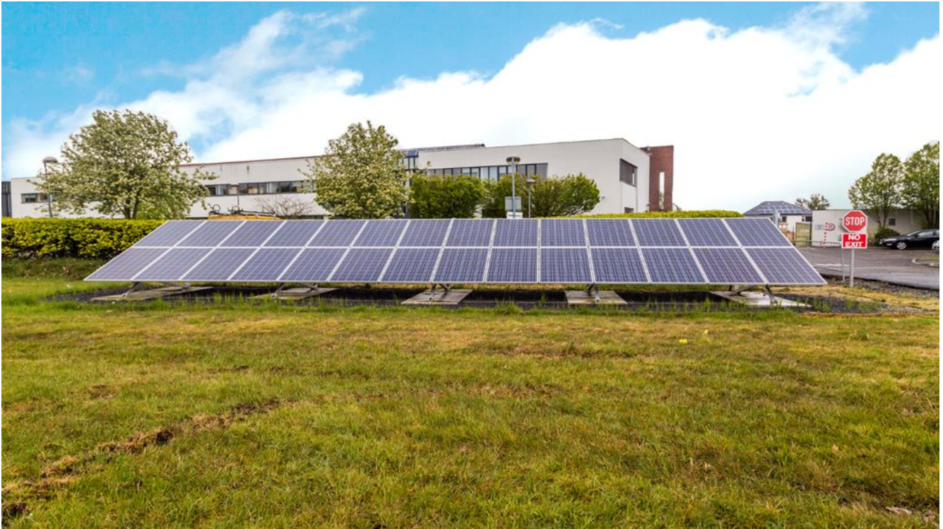
FIGURE 1: SOLAR PV ARRAY TRIAL SITE, PORTLAOISE, CO. LAOIS
