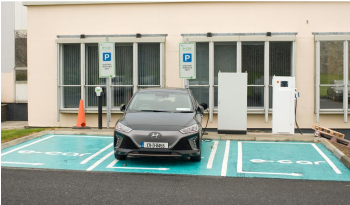
Figure 1: EV Charging Unit containing SUCCESS components, Leopardstown Road, Dublin
