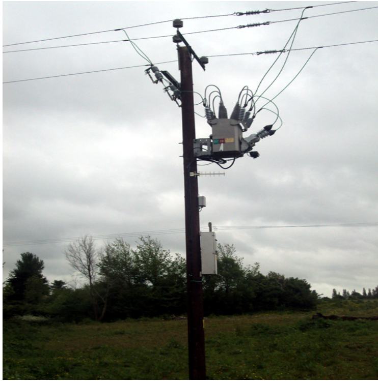
Figure 1 MV Pole Mounted Recloser
