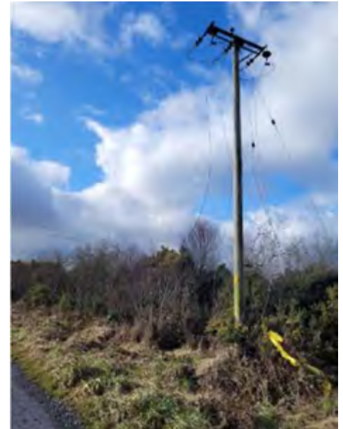
Third Party Damage causing grounded electricity line
