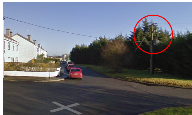
Figure 5 Pole mounted three phase 100kVA transformer feeding three-phase LV line from which single-phase circuits are extended to each house
