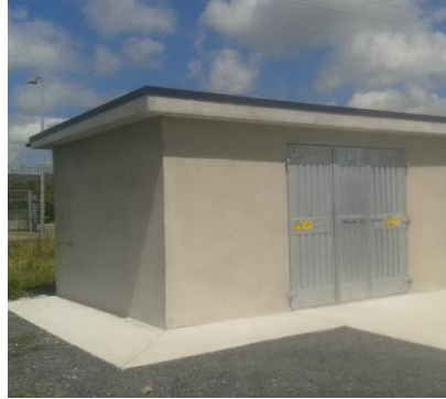
Fig. 1: Freestanding MV substation.
