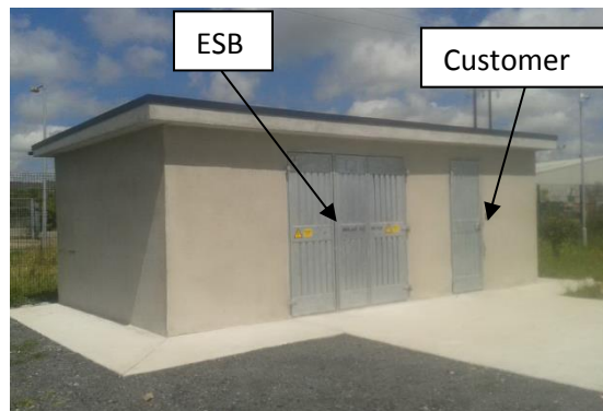
Fig. 2: Freestanding MV substation adjoining a customer's switchroom.
