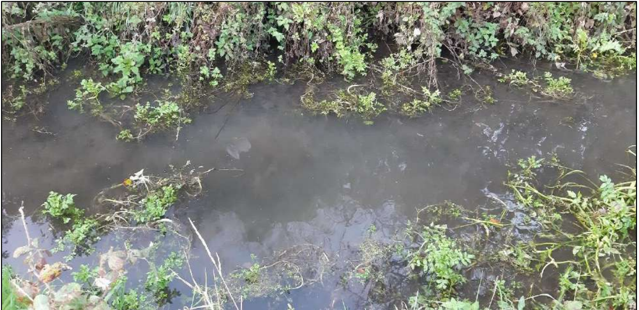
Photo 6: Image of nearest drainage channel, north of leak point, showing the poor water quality and stagnant water observed.
