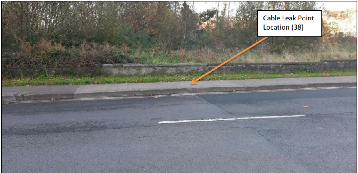
Photo 1: View north from Monaghan Road looking into section of concrete pathway that is associated with the leak point. Cable progresses north and west from this point. Note green area in background extends for c.50m to north where drainage channel is located.
