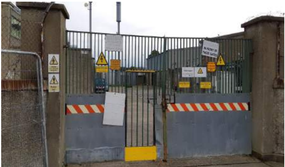
Photo 10: Entrance to substation at end of laneway. Concrete yard with gravel areas. Substation is circa. 200m northeast of recorded leak point
