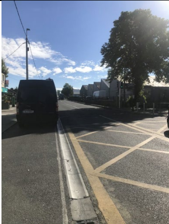
14-05 – Road surfacing in generally good condition on Sallynoggin Road. With shallow surface water runoff drainage channels.
