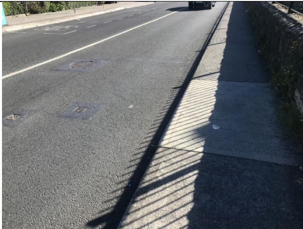
14-01 – Different concrete present at indicative leak location, suggesting more recent works in that area.
