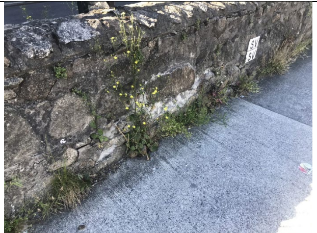
14-02 – Damage / repair works to wall adjacent to indicative leak location.
