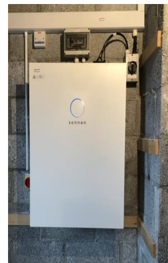
FIGURE 6 - RESIDENTIAL SCALE BATTERY
