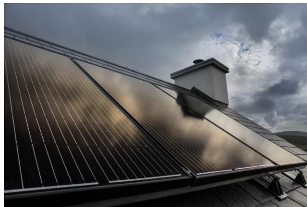
FIGURE 13 – SOLAR PV INSTALLATION
