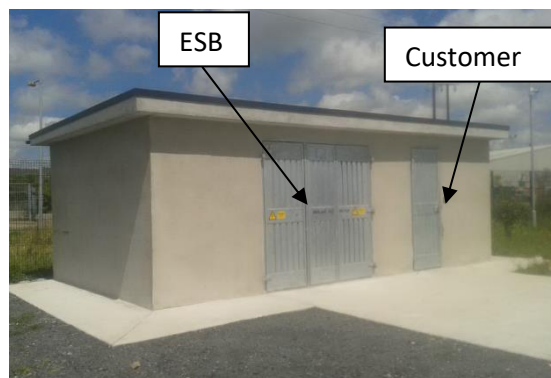
Fig. 2: Freestanding MV substation adjoining a customer's switchroom.
